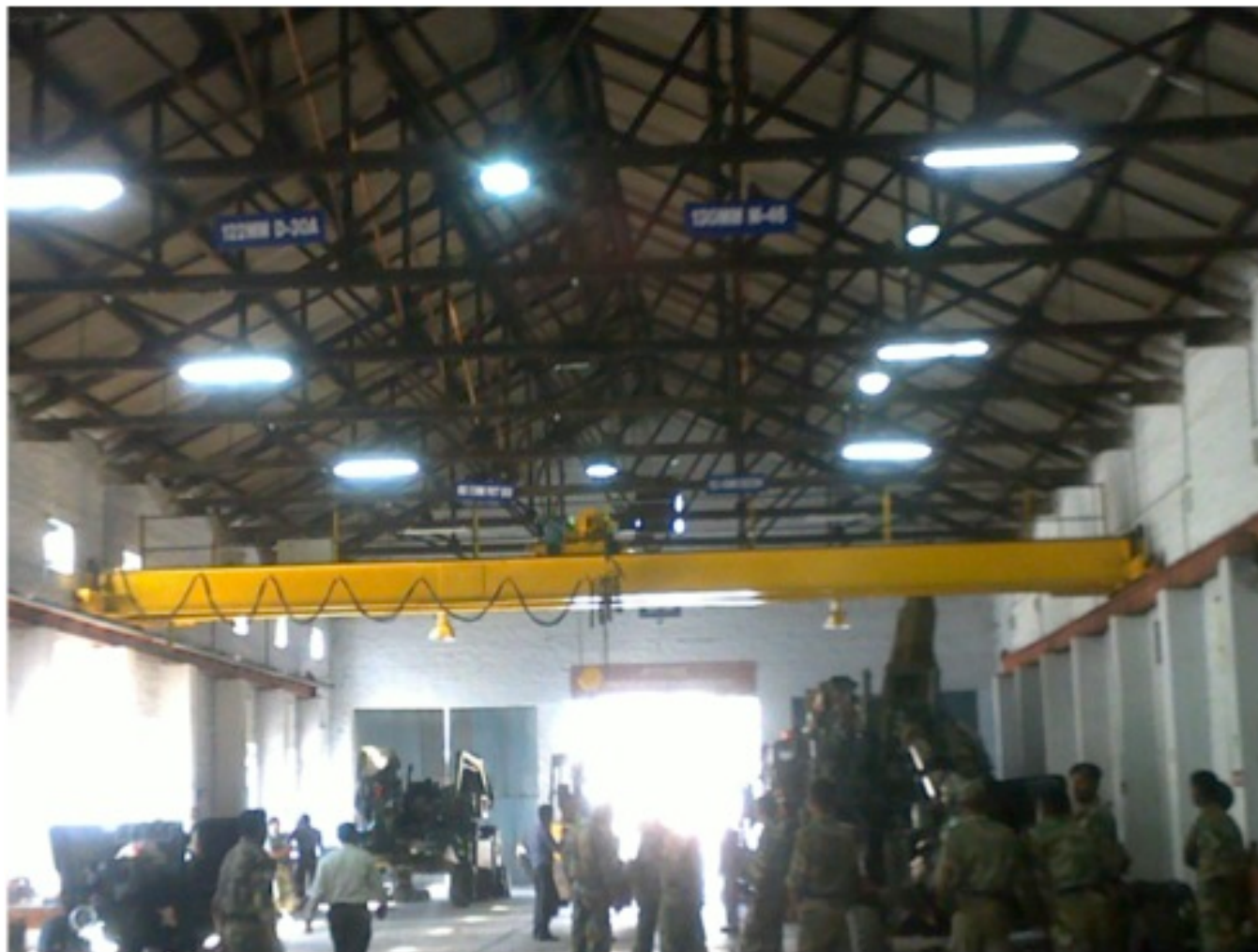
15T EOT Crane at 506, Army Base Workshop, Jabalpur
